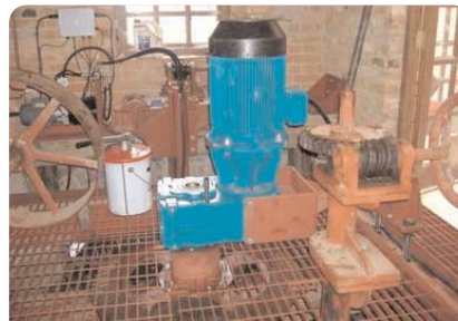
Plant room for a 10 kW micro hydro scheme
