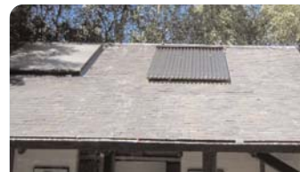
2m 2 of evacuated tube collectors
